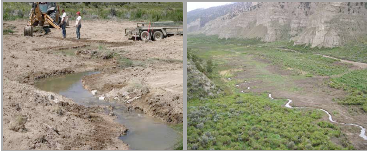
These photos show a stream-channel realignment project that improved water quality and wildlife habitat in Piute County.
